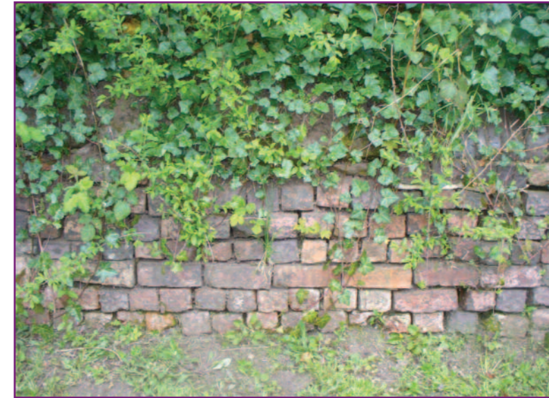
Old brick wall retaining the bank beside the towpath as the canal descends in a cutting
