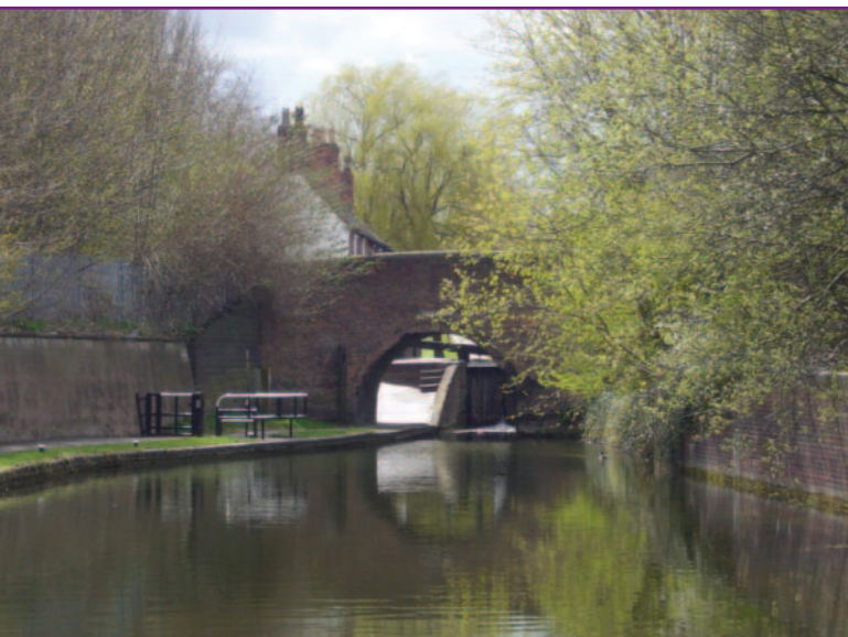
Looking south towards Top Lock. Note the motorcycle barriers and mooring bollards on the towpath.
