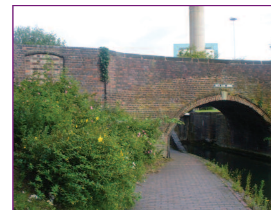
Fox's Lane Bridge is one of the classic elliptical brick bridges of the BCN. On the left is an in-filled gateway that once controlled access to the towpath.
