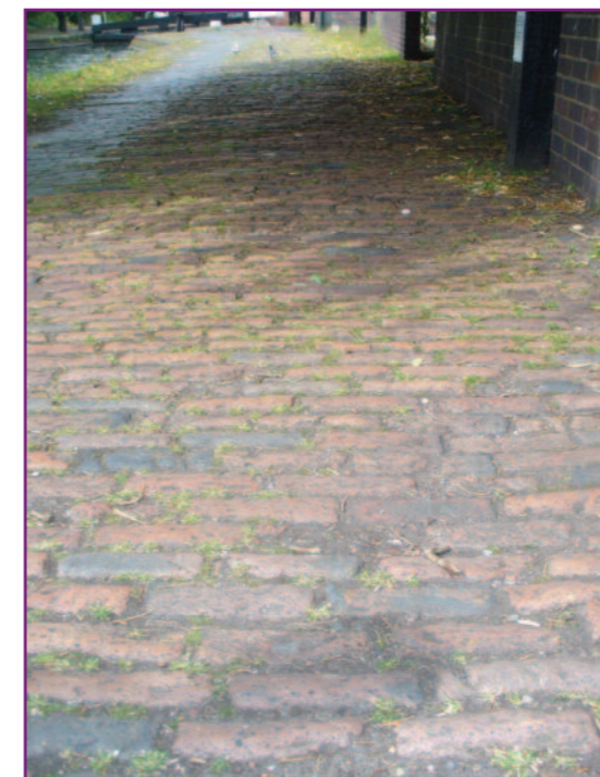
Worn and patched paving at Top Lock.
