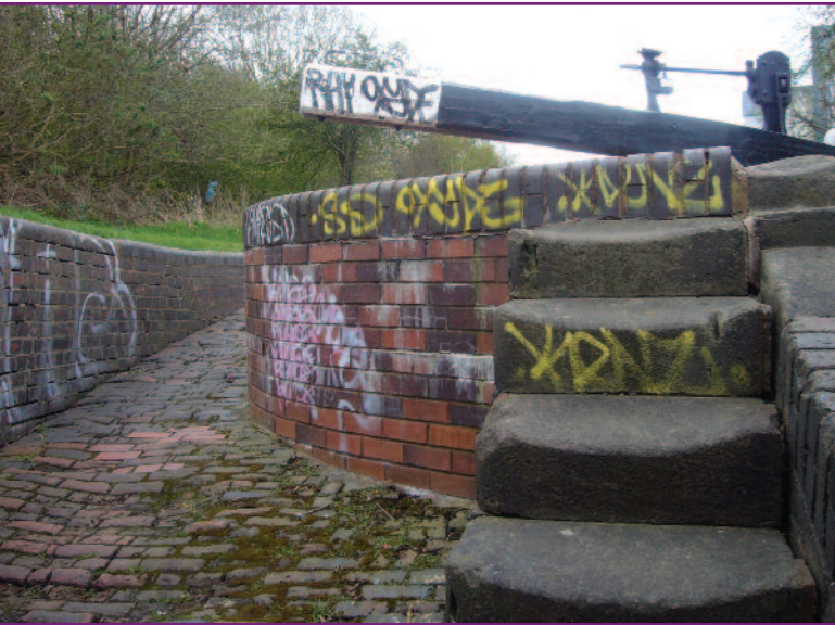
Canal area that has been defaced and spoilt through illegal graffiti activity.
