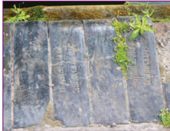
Bull nosed brick copings to the canal wall with the impressed makers name of Whitehouse Bloomfield.
