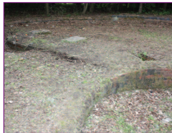
Remains of the railway turntable in Fowlers Park are of archaeological significance.
