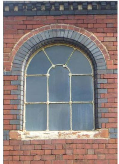
Detail of the Crown Nail Works building including locally manufactured wire cut and moulded brick, colour contrast brick detailing and iron framed window.
