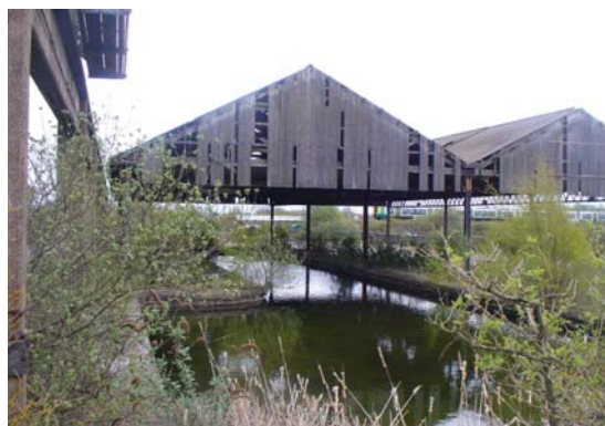
Chillington Wharf is the last of some 30 similar canal rail interchanges on the BCN retaining evidence of all the stages of its development. It recognised as a nationally significant heritage asset for its historical and technological interest, intactness and rarity.
