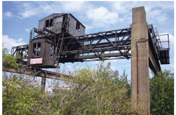
The 1930s travelling crane at Chillington Wharf is part of the grade II listed structure.
