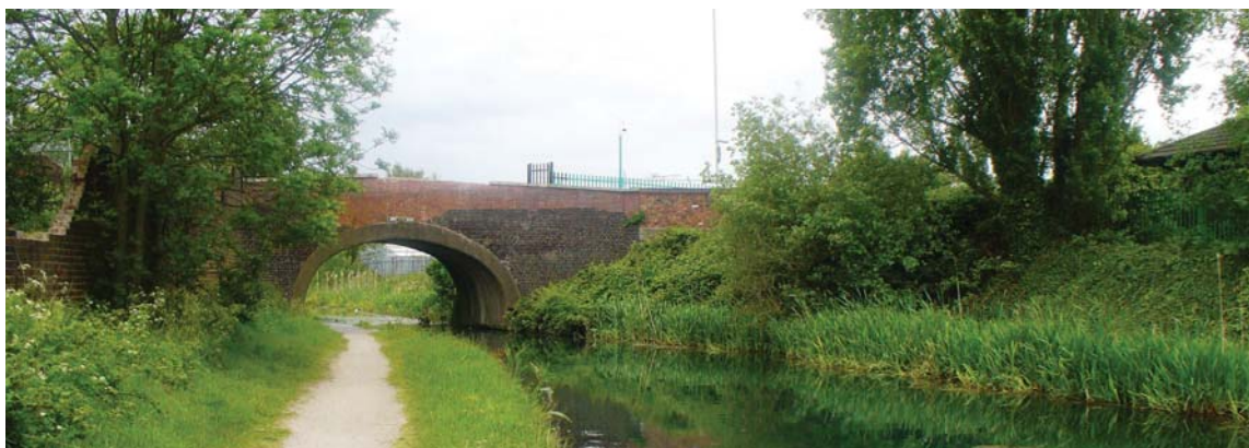
Jibbet Lane Bridge – one of a series of historic bridges along the canal. Whilst altered this bridge retains much original fabric.
