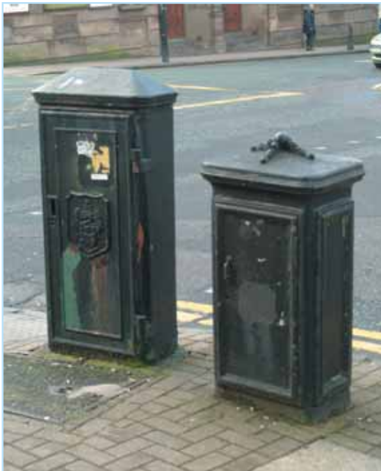
Above: Electricity distribution cabinets. Right, early cabinet possibly associated with the Lorain tram system. Left, Margery style cabinet.
