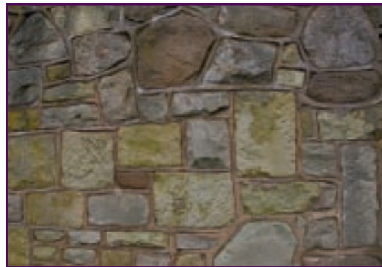
Above: Strap pointing to boundary walls
