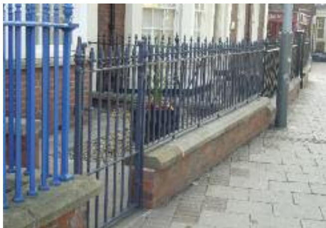
Railings and gates reinstated under the Townscape Heritage Initiative are protected by the Article 4(1) Direction.
