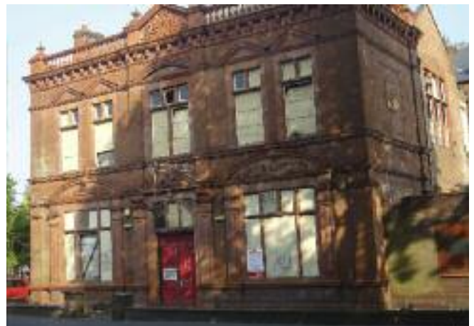
The vacant former Technical School is at risk of further deterioration as a result of its vacant condition.
