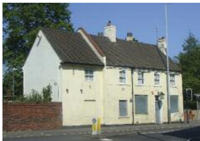
The former Swan Bank Tavern, Lichfield Street is one of a number of vacant buildings in Bilston at risk of deterioration.
