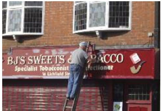
Regular maintenance is essential to protect historic features and the investment made under recent grant regimes.
